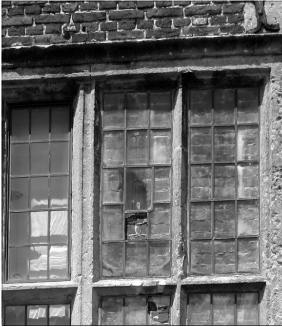
Fig. 7. Close up view of the window with the crude opening in the brickwork and slightly larger glass pane. The missing pane of glass just below, judging from very early photographs, has been missing for some time.
